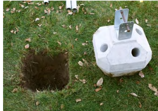
Figure 5. Tapered Hole for Concrete Head
